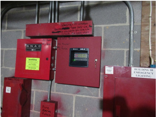
Control panel overview
