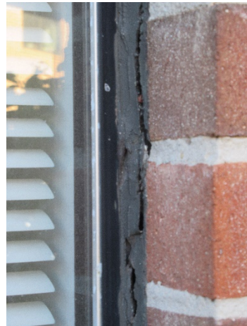
Sealant crack at building 88
