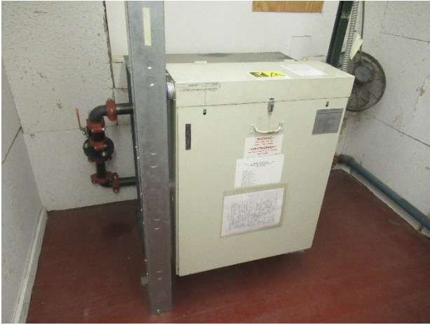
Elevator controls, 2001 replacement
