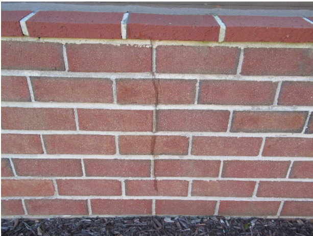
Masonry crack at building 88
