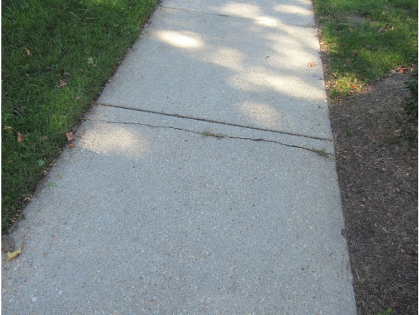
Concrete sidewalk crack
