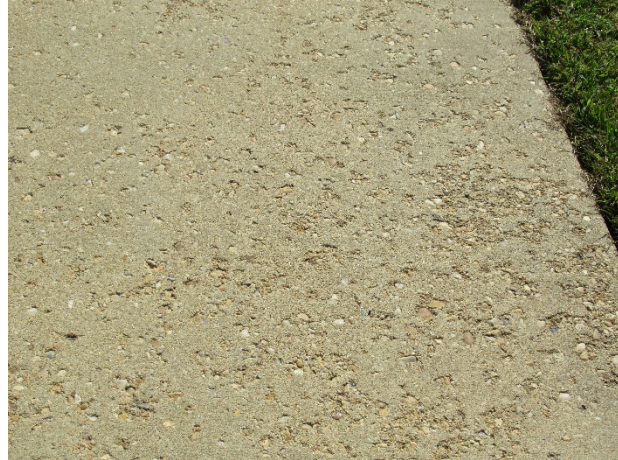
Concrete sidewalk scaling
