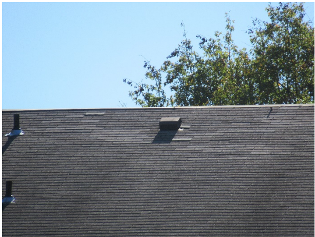
Isolated missing shingles
