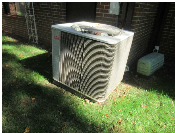
Air handling unit overview
