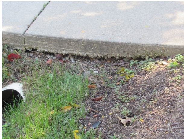
Concrete sidewalk undermining
