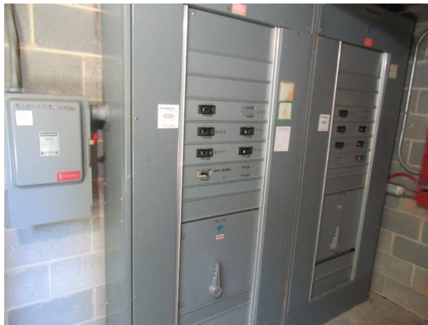
Electrical panel overview
