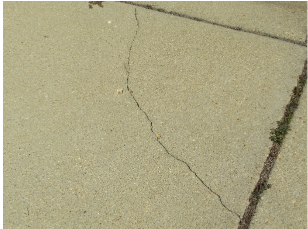
Concrete sidewalk crack
