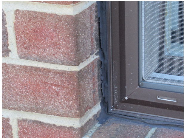
Sealant cracks at building 92
