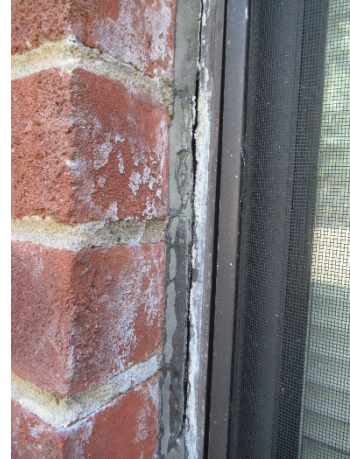
Efflorescence and sealant deterioration at building 94
