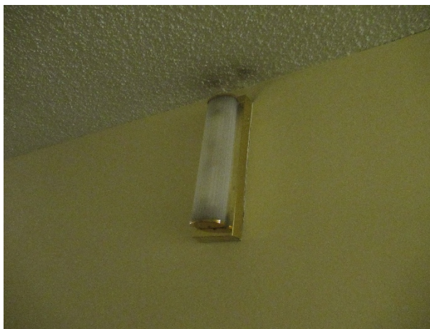
Finish deterioration and burnt out bulb
