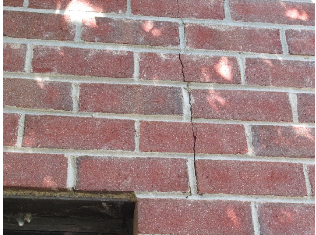
Masonry and mortar cracks at building 92
