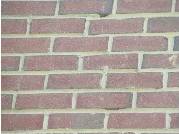
Mortar deterioration at building 89
