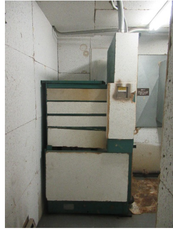
Elevator controls, original
