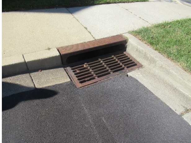
Catch basin overview
