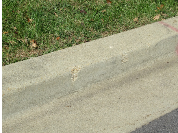
Isolated concrete spall
