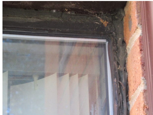
Sealant deterioration at building 93
