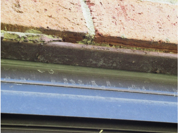
Lintel rust and mortar deterioration at building 93
