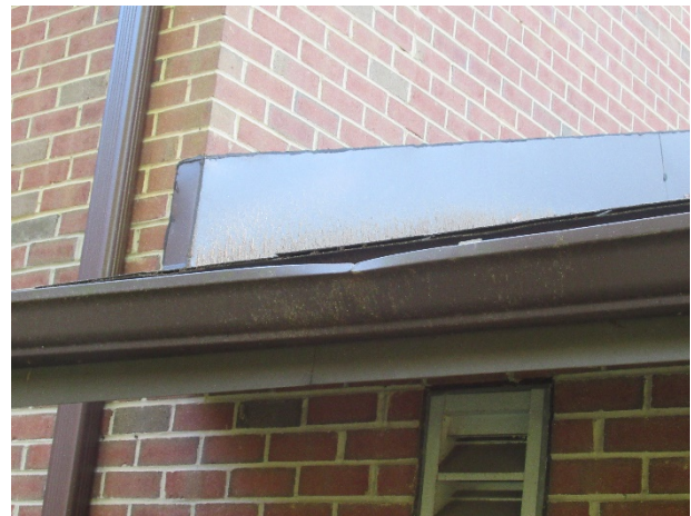
Isolated gutter damage
