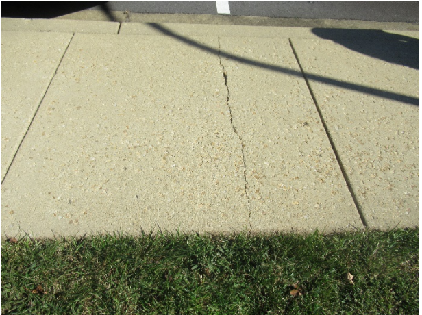
Concrete scaling and crack
