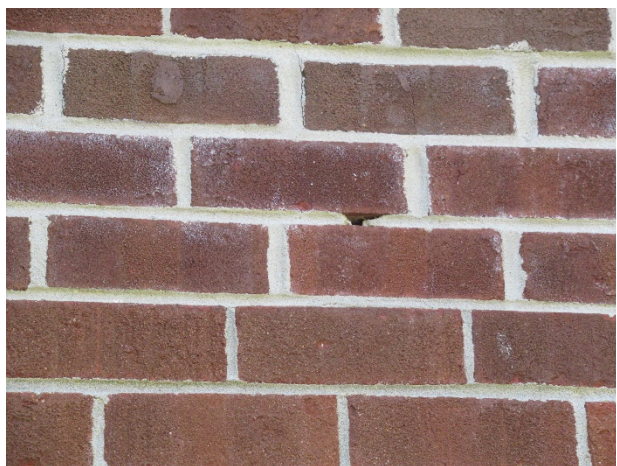
Efflorescence and mortar deterioration at building 90
