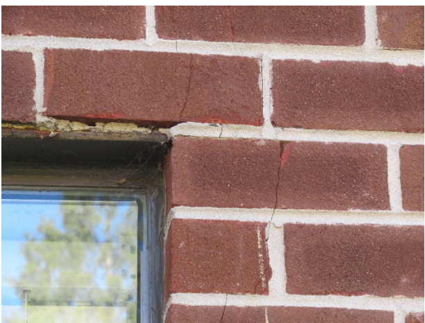
Masonry cracks and mortar deterioration at building 90
