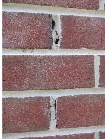
Efflorescence and mortar deterioration at building 88
