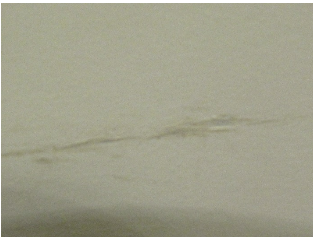
Scuff mark and damage
