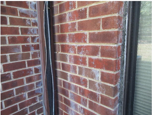
Efflorescence at building 94
