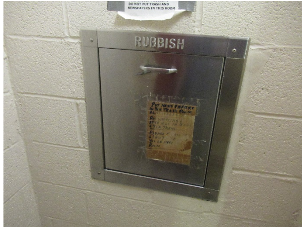
Trash chute overview
