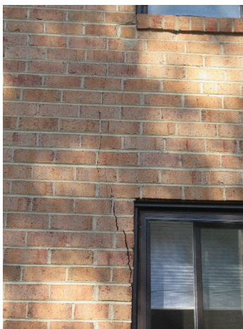
Crack at Building 93
