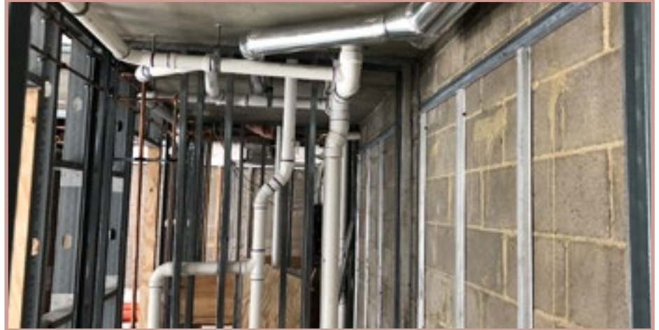
Rough-in work for plumbing, electricity and other utilities is currently underway in Building 91. Construction photos courtesy of Minkoff
